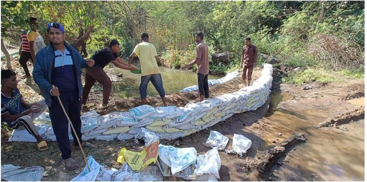
NSS volunteers creating bund in Ulhas river at Vangani to block the water for helping the villagers in water conservation as a part of the Rural Development Camp at Vangani, Dist. Thane of Maharashtra. (24 th to 30 th December, 2022)
